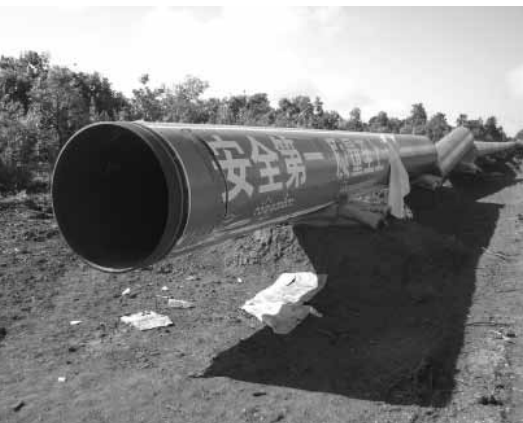
Pipeline to take Shwe gas to China Photo tab
