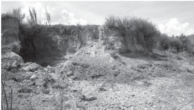
Erosion along the river banks due to a strong river flow in the rainy season
