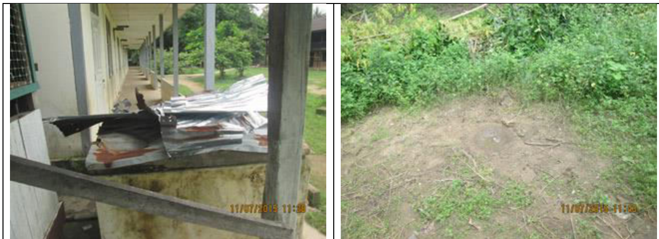
These photos were taken by a KHRG community member on July 11 th 2015, in Kawkareik Town, Kawkareik Township, Dooplaya District. The first photo shows a section of roof that was damaged when a grenade fired by DKBA soldiers from an M79 grenade launcher hit the primary school building in Chaung Taung section. The second photo shows where another grenade fired from the M79 grenade launcher hit the ground and exploded within the school grounds. No students were injured by either grenade. [Photos: KHRG]
