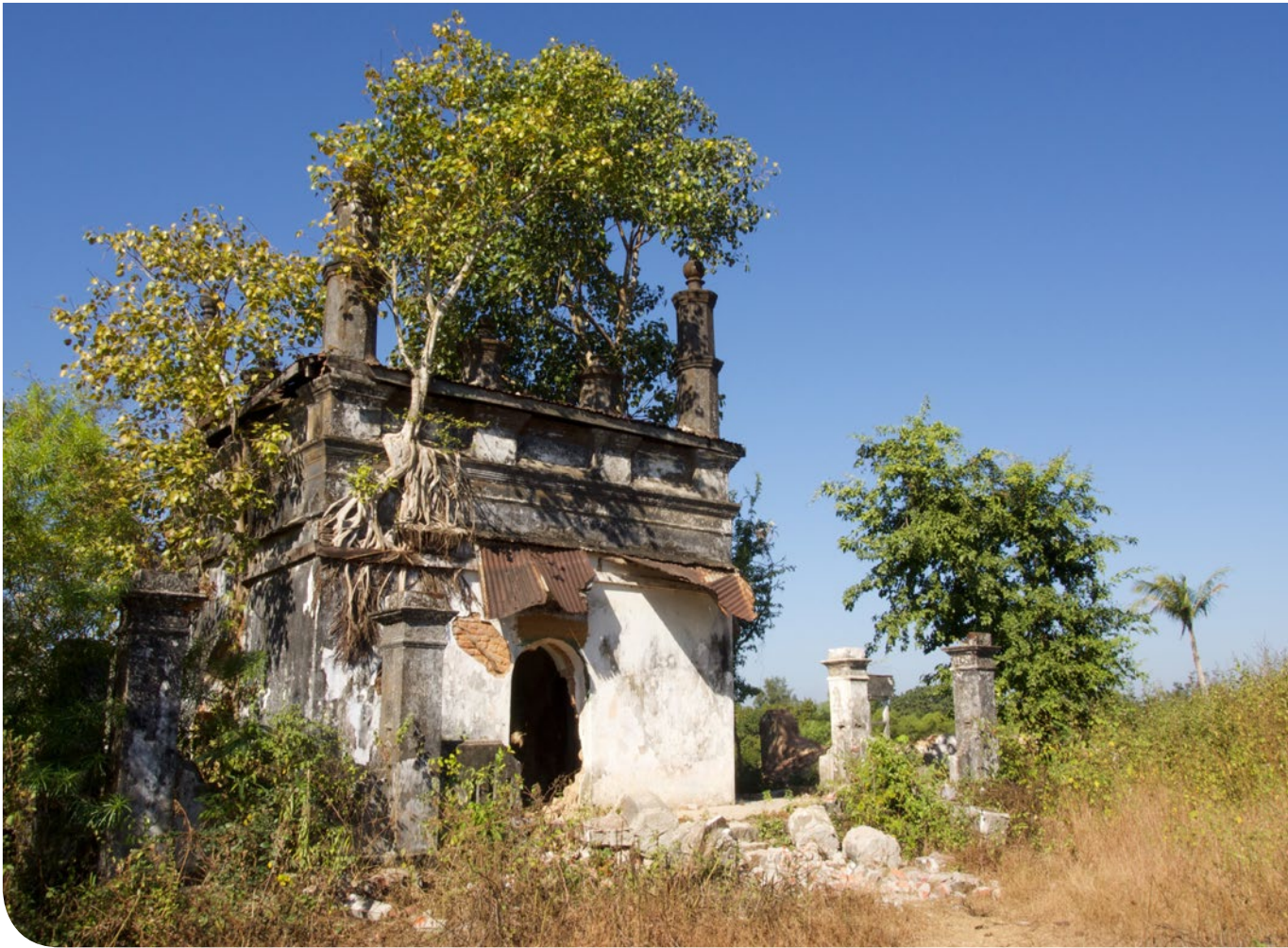
Mosque fallen into disrepair, outskirts of Sittwe, November 2014
