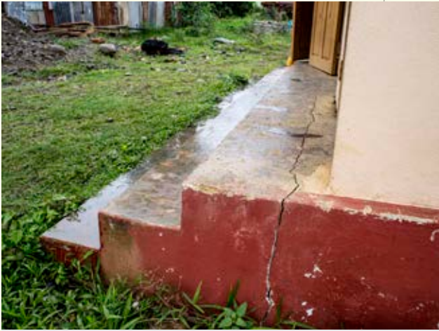
Cracks in one of the Kaday monastery buildings which the monks blame on the violence of the jade mining operations in the crater below. CREDIT: Minzayar
