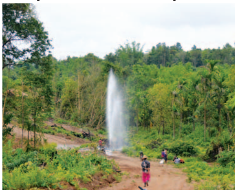
The pipe burst due to a build-up of pressure
