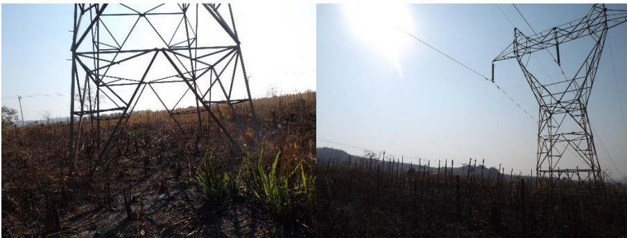
Electrical hubs outside Military Battalion 360 (Daw HsoShay) (photographs taken 25 February 2015).
