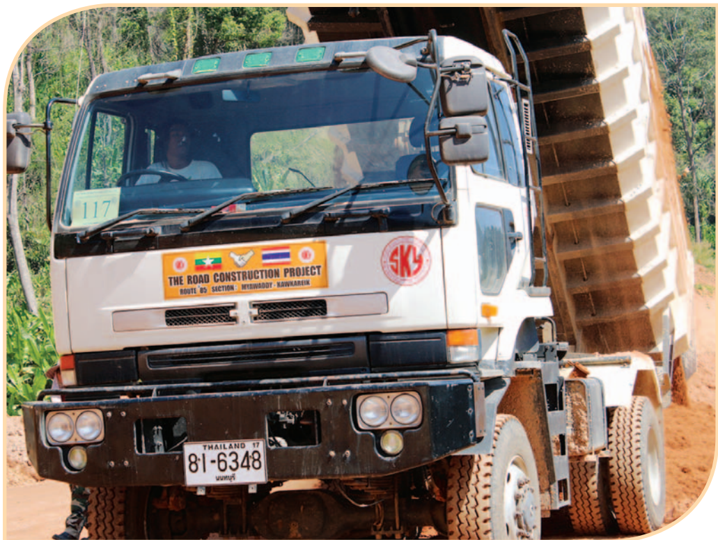
Construction truck on the Asia Highway road link from Thin Gan Nyi Naung to Kawkareik [Photo credit : KESAN]
