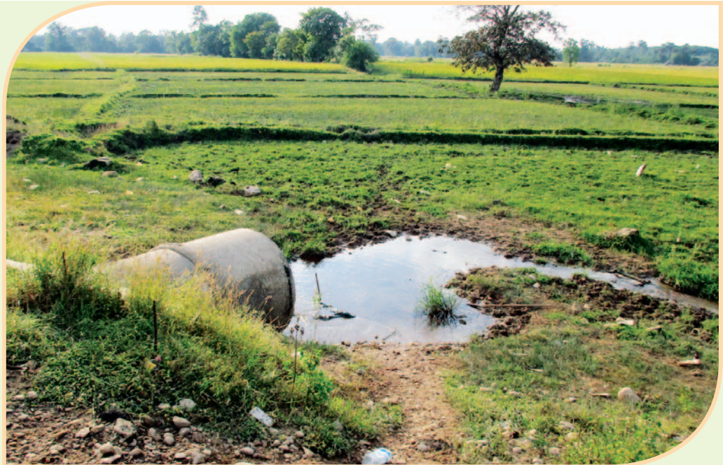
This photo was taken on 24th October 2015 beside the Asian Highway in Kawkareik Township. The photo shows the pipe that was built to allow run-off water from the road to flow into the paddy field. [Photo credit : KHRG]
